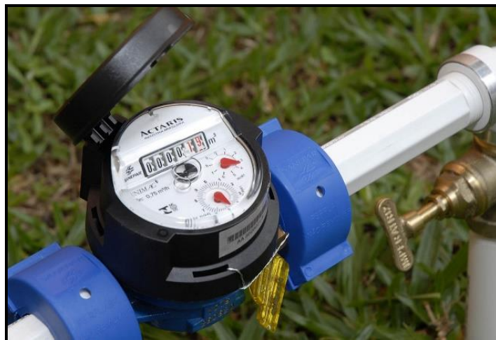
Figure 7 – Sanepar's standard water meter
