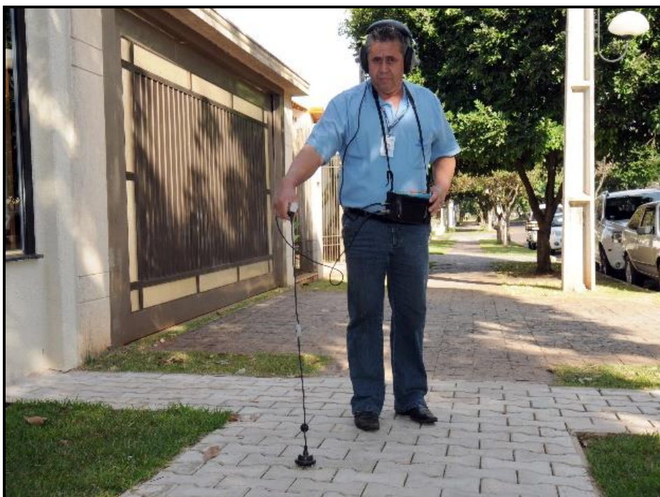
Figure 6 – Detection of leakages with the aid of the geophone
