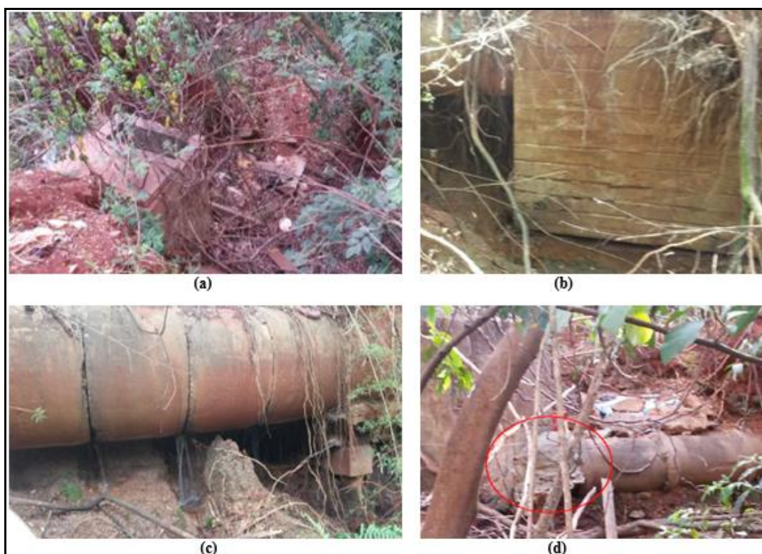
Figure 3 – Current state of the drainage system downstream of the park Alfredo Werner Nyffler
