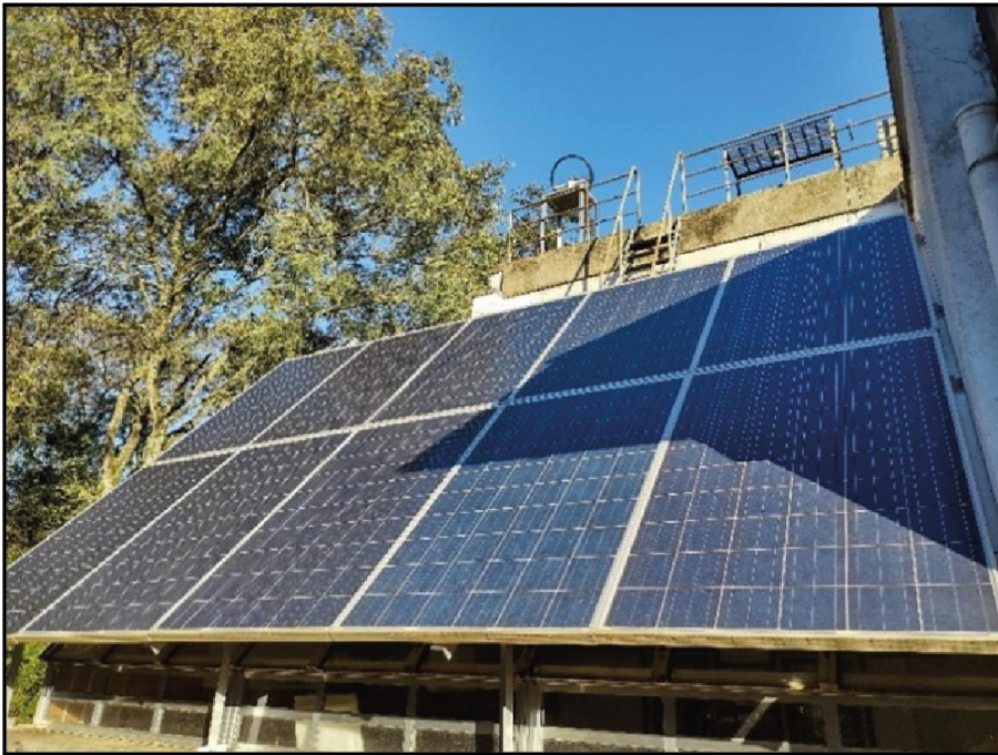
Figure 1 – Photovoltaic system installed at the Solar Energy Laboratory in Porto Alegre (UFRGS)
