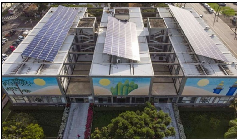
Figure 1 – Photo of photovoltaic panels installed at the headquarters of the City Hall of Curitiba
