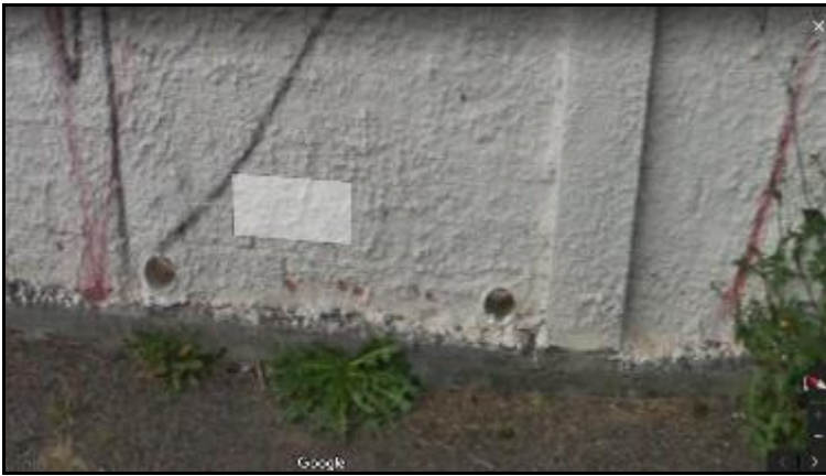
Figure 7 – Location where necrochorume is leaked
